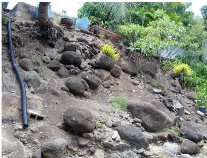
Figure 2: Corrugated pipe running from residence to channel along Wailupe stream and planting along bank, perhaps to prevent more erosion.
