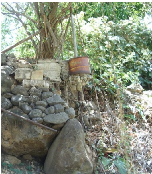
Figure 4: Severe Erosion along Wailupe Stream. erosion was a threat to property in this picture. The ban was eroded away from fencing on the property.
