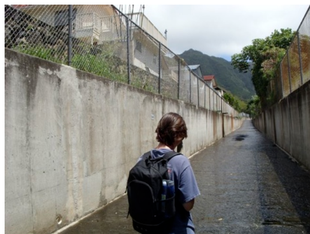
Figure 11: Upper reaches of Kuliouou channel, with vertical banks (no quick exist), and pipes from residence in connected to channel. Surveys of the upper reaches are not recommended.
