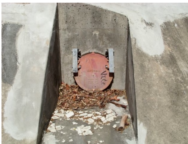
Figure 16: Storm water gate that opens into Kuliouou channel. Many were partially blocked by sediments and plant debris.
