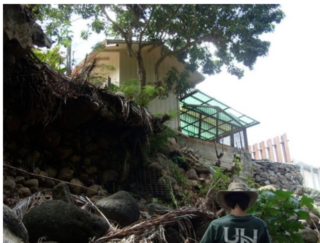
Figure 5: Bank undercutting along Wailupe stream, an example of severe erosion.
