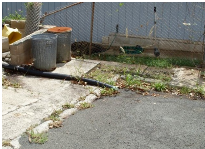
Figure 18: Corragated pipe running from residence to street, with a storm drain less than 20 feet away from the pipe. It wwas not clear what the resident was draining.
