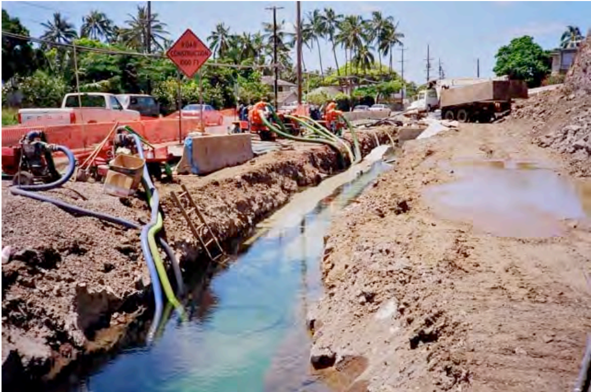
Figure 7. Water being pumped from flooded utility corridor during the Kalanianaʻole Highway widening project, ca. 1993. Photo: T. Hara, courtesy MFHC.
