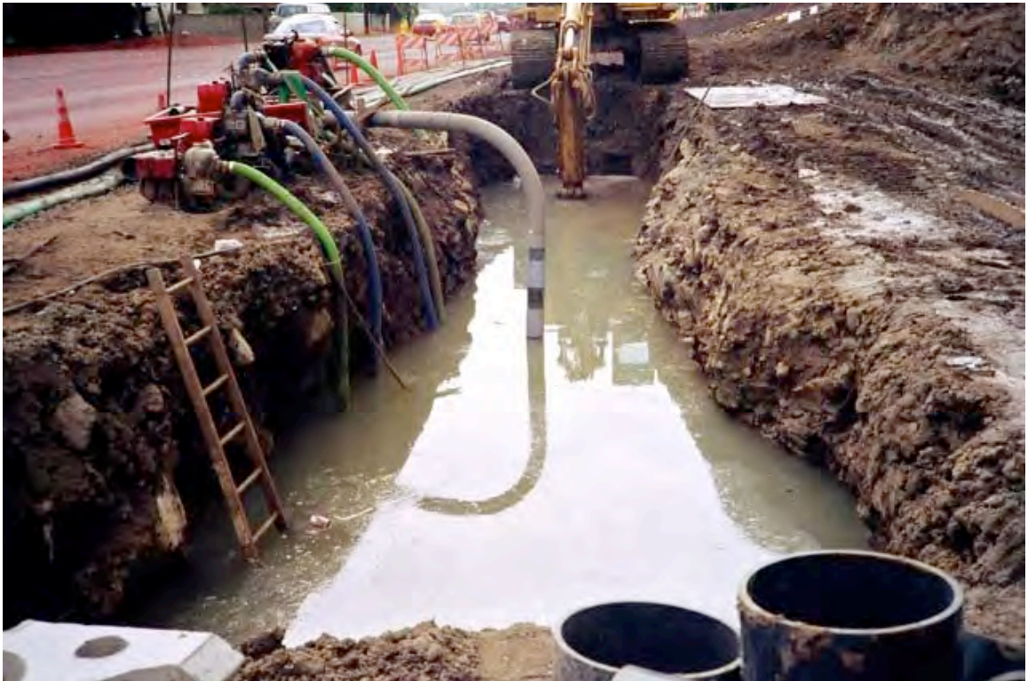
Figure 6. Water being pumped from flooded construction site landward of the Lucas Spring Study Site, ca. 1993. Photo: T. Hara, courtesy MFHC.
