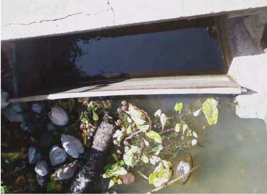
Figure 16. Plywood barrier separating Kanewai Fishpond (bottom) from Paiko Lagoon (top). Photo: J Kennedy.
