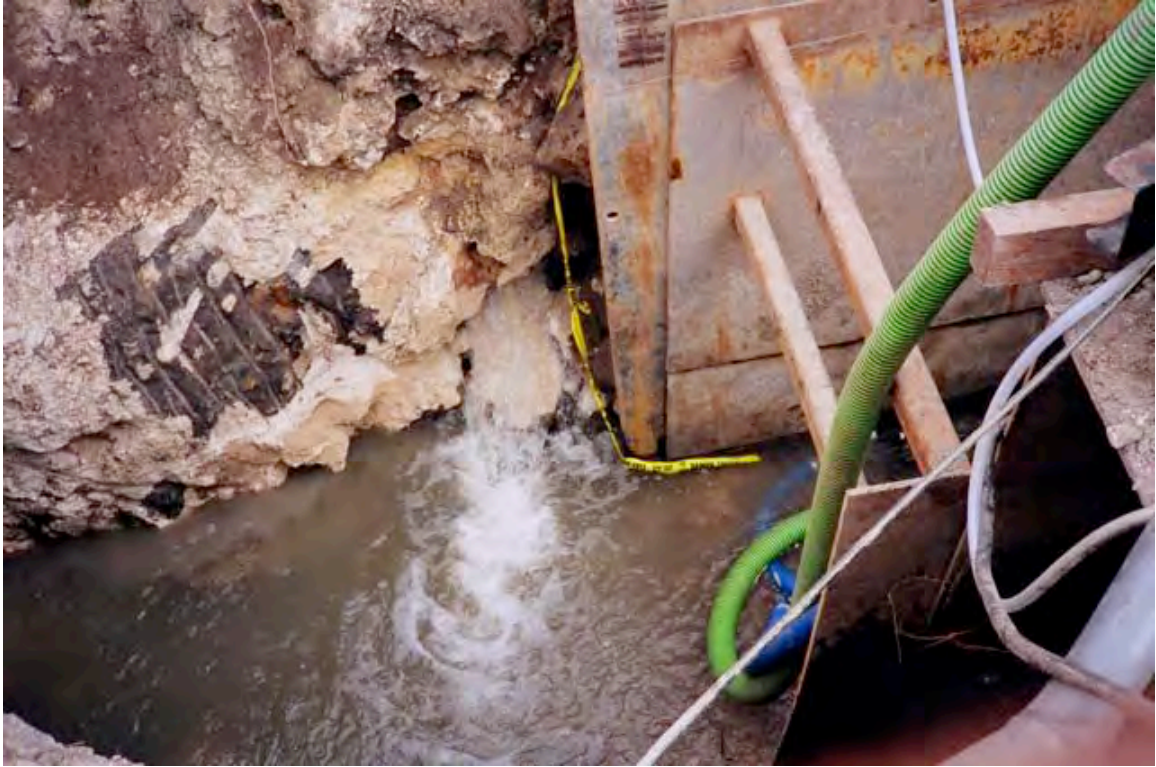
Figure 5. Water flowing out of probable broken lava tube conduit during the Kalaniana'ole Highway widening project, ca. 1993. Photo: T. Hara, courtesy MFHC.
