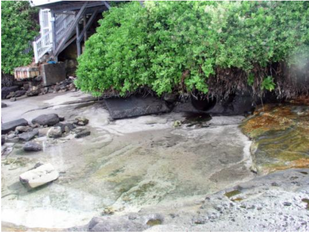
Figure 2. Drainage outfall and headwall fronted by limestone bench and water filled depressions at Project site.
